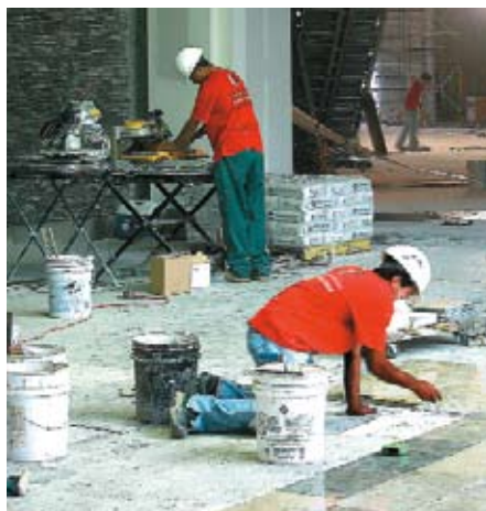
Mer-Krete’s 750 Rapid-Setting Thin-Set mortar meant grouting could begin quickly. A custom-made version of 211 Thin-Set mortar provided installers with the proper, thick bed to evenly support the troublesome sizes and thicknesses of the stone tiles.
